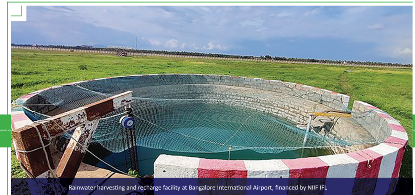
Rainwater harvesting and recharge facility at Bangalore International Airport, financed by NIIF IFL
